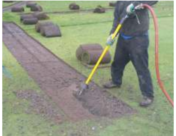
Air Spade utilized to pulverize soils and construct bunkers for new root zones.
