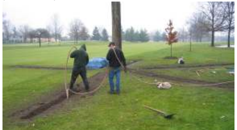
Five bunkers, to be back filled with amendments; all done in half a day
